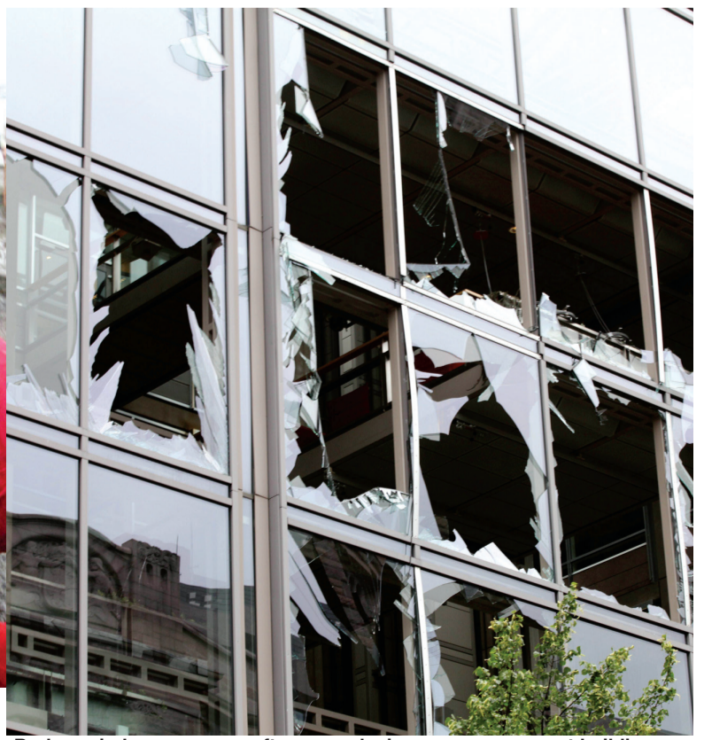
Broken windows are seen after an explosion near government buildings in Norway's capital Oslo -AFP
