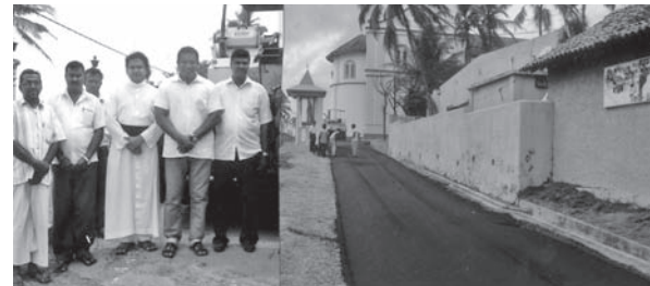
Western Provincial Councillor Al Haj M.M.M. Amjad and Rev. Fr. Nisantha Perera, Parish Priest Polkotuwa being conducted to the road, under construction, under the "Maga Neguma" program at St. Anne's Road, Polkotuwa, Beruwala recently.
