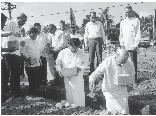
The foundation stone was laid by the Water Supply and Drainage Minister Dinesh Gunawardane and the Provincial Minister Upali Kodikara for the proposed supermarket complex of the Maharagama M.P.C.S. at Udahamulla recently. Pic: Wehelle Piyathilake, Maharagama Spl. Cor.
