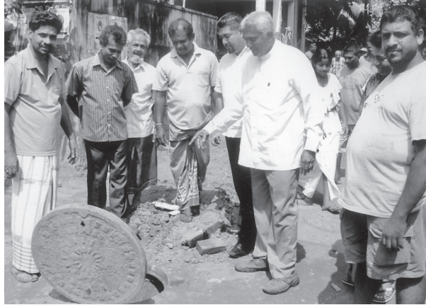
Western Provincial Councillor and Founder of Pragna Pradeepa concept, Jayantha de Silva who was instrumental in the laying of new pipelines along Kent Road, Dematagoda paid a visit to the area recently. Here Silva inspects a manhole.
