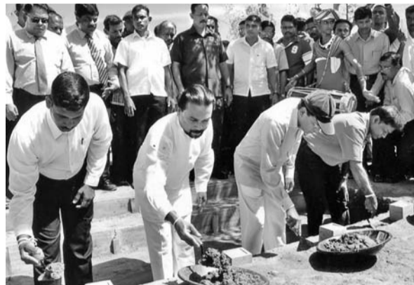
The foundation stone for the Viru Upahara housing project at Mahasenpura, Polonnaruwa was laid under the patronage of Construction, Engineering Services, Housing and Common Amenities Minister Wimal Weerawansa and Health Minister Maithripala Sirisena recently. The project to be launched under the Janasewana one million housing program is estimated to cost Rs. 6 million and benefit 30 terrorist-hit families. Colombo District MP Thilanga Sumathipala, Construction Ministry Secretary P.H.L. Wimalasiri Perera and NHDA General Manager Brig. Mahinda Mudalige were present. Pic: Ashraff.A.Samad,Dehiwala-Mt.Lavinia Spl.Cor.
