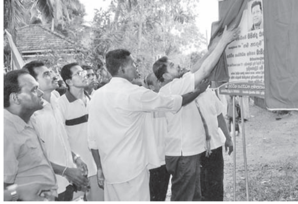
Indigasthuduwa Temple Road in Matugama was concreted at a cost of Rs. one million recently. Here the Western Provincial Councillor Chandrabanu Adikaram unveils the plaque. Pradeshiya Sabha member Sriyananda Wickremathanthri looks on.
