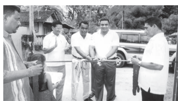
Western Provincial Councillor, M.M.M. Amjad opened the newly constructed road at Chamara Uyana, Payagala recently. Vice Chairman, Beruwala Pradeshiya Sabha, Kusman de Silva is also in the picture.
