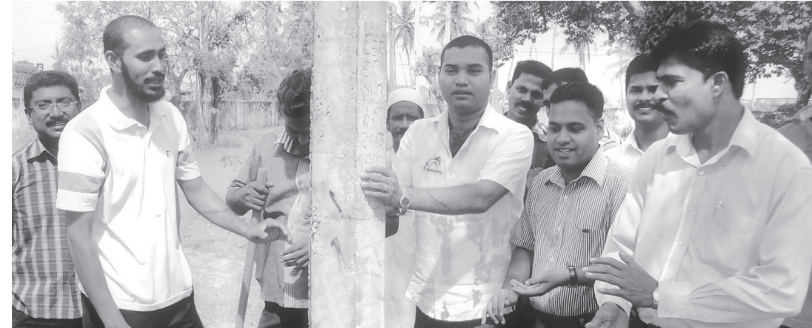
A new electricity project was commissioned by the Akkaraipattu Mayor, A. Ahamed Zackie at the Akkaraipattu Muslim Burial Grounds recently. Municipal Commissioner A.L.M. Azmi, Councillors N.M. Najimudeen, K.L.M. Zarook and A.L. Junaideen were also present. Pic: I.L.M. Rizan, Addalaichenai Central Cor.
