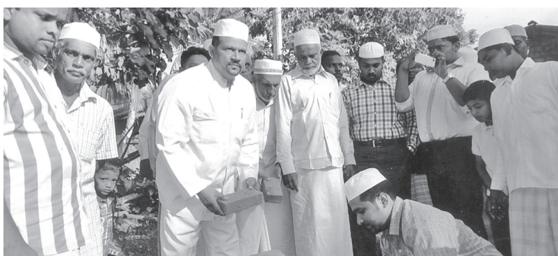
The foundation stone was laid for a new building at Najeeb Hajjiyar Education Centre, Dharga Town recently. Here Al Haj M. Najeeb Hajjiyar bin Ameen Alim lays the foundation stone. Pic: B.M. Mukhtar, Beruwala Spl. Cor.
