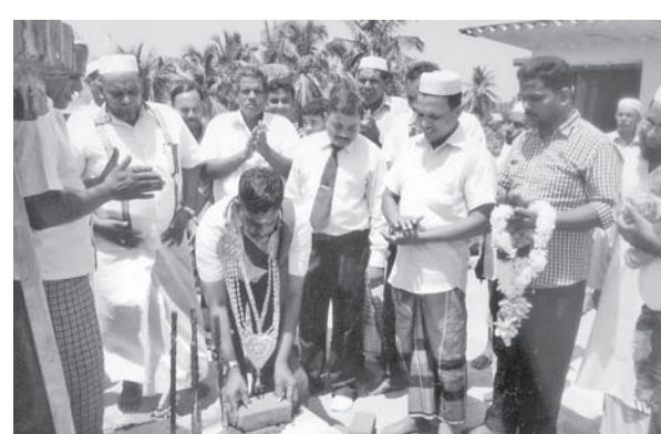
The foundation-laying ceremony for a 'Manarah' at the Masjidhul Saliheen Jummal Mosque, Maligaikadu was held recently. Here Digamadulla district parliamentarian, P.H. Piyasena lays the foundation stone.
