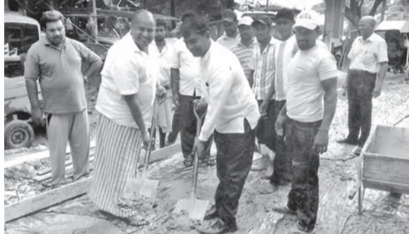
The M.H.M. Ashraff Road at Palavi Malihaapuram in Puttalam will be rehabilitated with concrete, with fund allocations from North Western Provincial Councillor, S.H.M. Niyas. Here work in progress.
