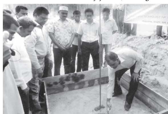
The foundation-laying ceremony for an information technology faculty complex at Zahira College, Kalmunai was held recently. Here Digamadulla district parliamentarian H.M.M. Harees lays the stone at the site. Eastern Provincial Councillor, A.M. Jameel, principal P.M.M. Badurdeen are also in the picture.
