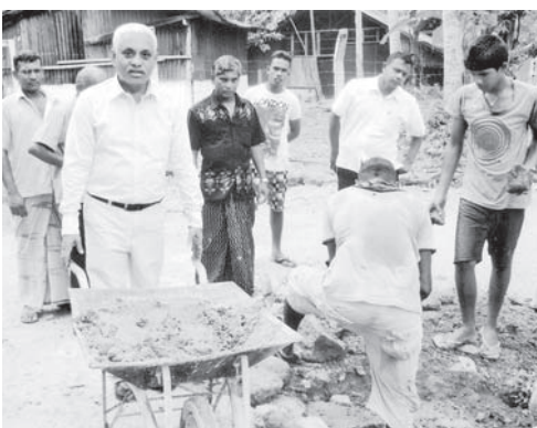
Parliamentarian Al-Haj M.S.M. Aslam takes part in the rehabilitation work on the road leading to Askvali Estate, Agalawatha recently.
