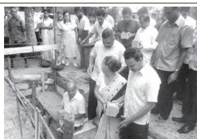
Chairman of the Panadura Urban Council Nandana Gunathilleka lays the foundation stone at Y.S. Obert Silva Mawatha at Nalluruwa, Panadura for a clinic and a public library. The land valued at Rs. 3 million was donated to the Panadura Urban Council by Mrs. Herath, sister of the late Ven. Panadure Ariyadamma Thera. Western Provincial Councillor Ranaviru Vikum Gunasekera also participated.
