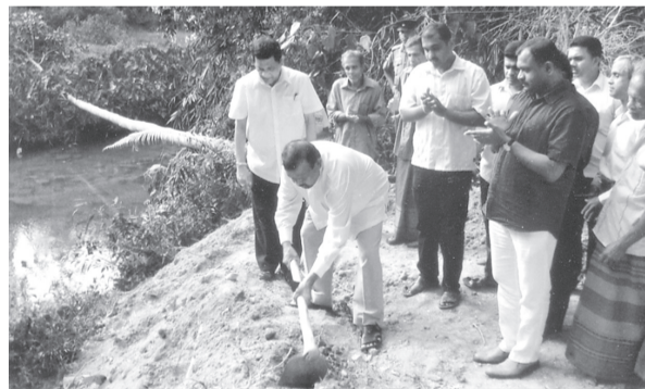
The foundation stone for a bridge across Kadiran-dola on the Dangala-Banagala Road in Pitabeddara Pradeshiya Sabha area was laid recently. Here Deputy Minister of Economic Development S.M. Chandrasena cuts the first sod. Deputy Minister of Public Administration, Wijaya Dahanayake is also in the picture.
