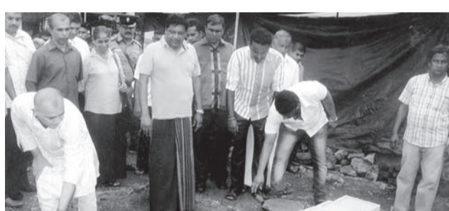
A shopping complex constructed at a cost of Rs. 500 lakhs will be built in Mathugama in the near future. Here Local Government and Provincial Councils Minister A.L.M. Athaula and Western Provincial Councillor Senal Welgama lays the foundation stone. Transport Minister Kumara Welgama is also in the picture. Pic. M.S.M. Munthasir, Panadura Central Gr. Cor.
